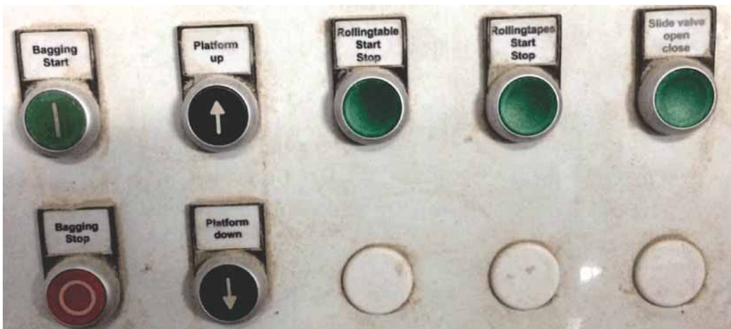
Figure 7-30: Control elements of the bagging unit
